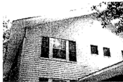
Artificial siding added to this house has altered the relationship of the window moldings to the exterior wall, and the house has lost details.
