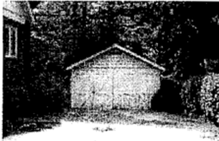
This wood-framed garage is a historic feature of this property and should be retained.
