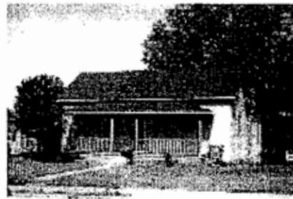
This saddlebag house has lost its central chimney, an important character-defining feature of the saddlebag house type.
