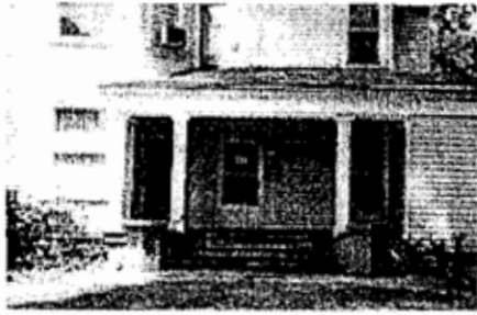
The original entrance door has been replaced with a new wood door and storm door, both of incompatible design.
