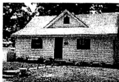
This once open front porch has been completely enclosed as an interior space, drastically altering the house's front facade.
