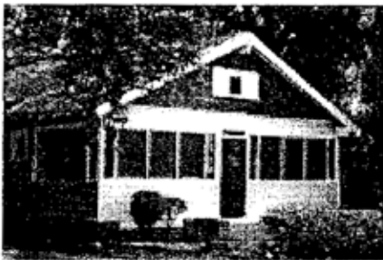
This front porch has been partially enclosed with screen and partially with solid siding. Enclosing it only with screen would have retained more of the original open feeling.
