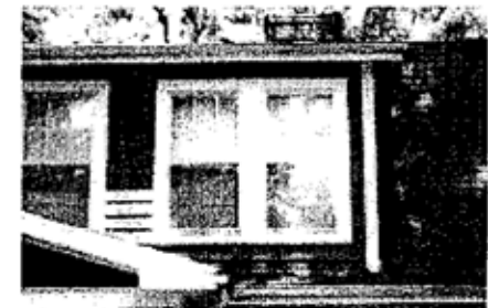
These storm windows are removable and do not detract from the historic window pattern.
