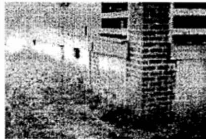
This brick pier foundation has been inappropriately infilled with concrete blocks.
