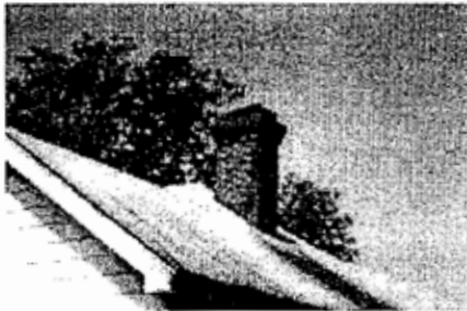
This corbeled brick chimney is an important feature and should be maintained.
