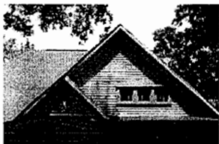
This decorative gable is an important character-defining feature of this turn-of-the-century house and should be maintained.
