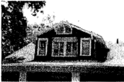
This gabled roof with dormer is an important character-defining feature of this house, and the visible roof form should not be altered.
