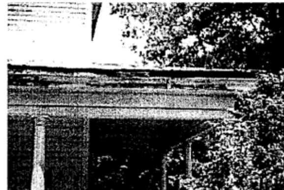
Lack of maintenance of a house's features and materials leads to deterioration.
