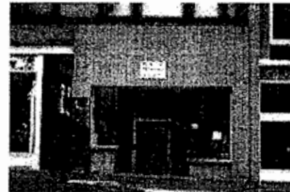
Incompatible vertical wood siding has been applied to this storefront.
