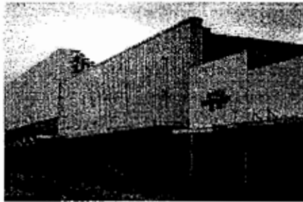
Incompatible coverings on upper facades.
